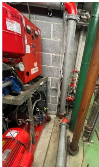
Figure 2: Existing Diesel/Electric Hydrant pump
