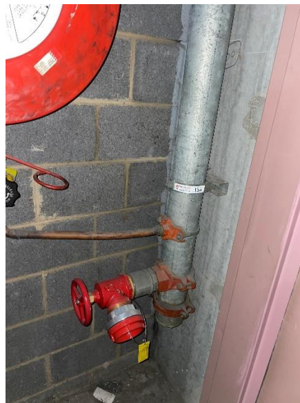
Figure 4: Fire hydrant in cupboard.
