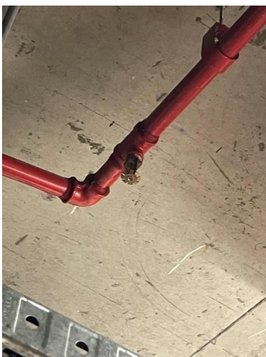
Figure 7: Sprinkler heads example and sprinkler pipes
