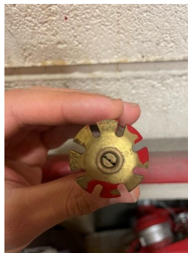
Figure 8: Sprinkler heads example and sprinkler pipes
