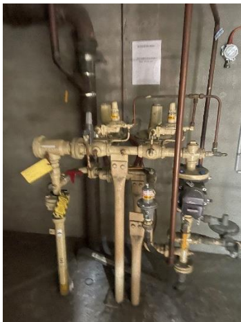
Existing High pressure gas boundary regulator.
