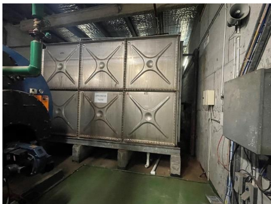
Figure 5: Roof top combined potable/fire hydrant tank.
