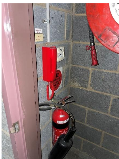
Figure 18: WIP/ECP points within cupboard.
