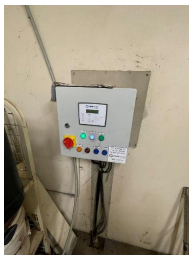
Existing Stormwater pumpstation control panel.
