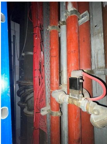
Figure 6: On-floor sprinkler control valve assembly
